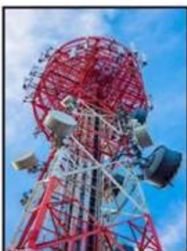
Self Supporting Tower (SST)
